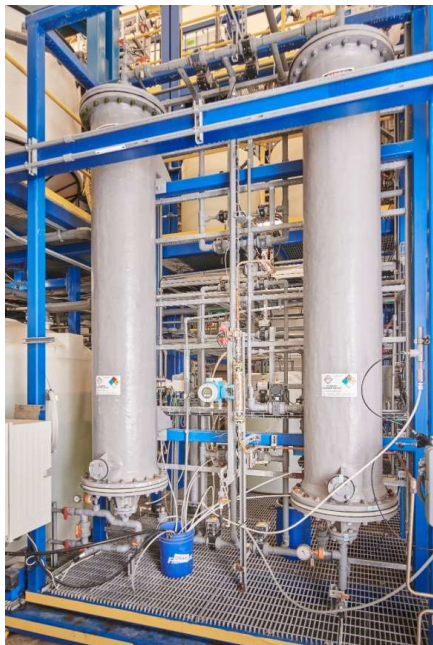
Figure 13-6: Calcium, Magnesium, and Boron Ion Exchange System at the Demonstration Plant
