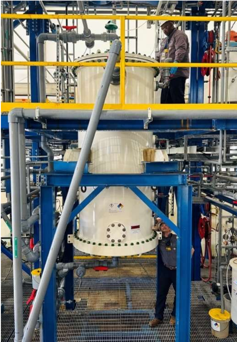
Figure 13-4: Commercial-Scale LSS Column at the Demonstration Plant
