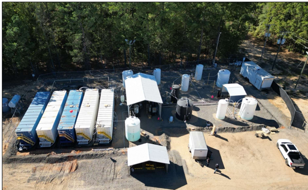
Figure 13-3: Temporary LSS Pilot Plant at the Mission Creek Dorcheat Gas Plant
