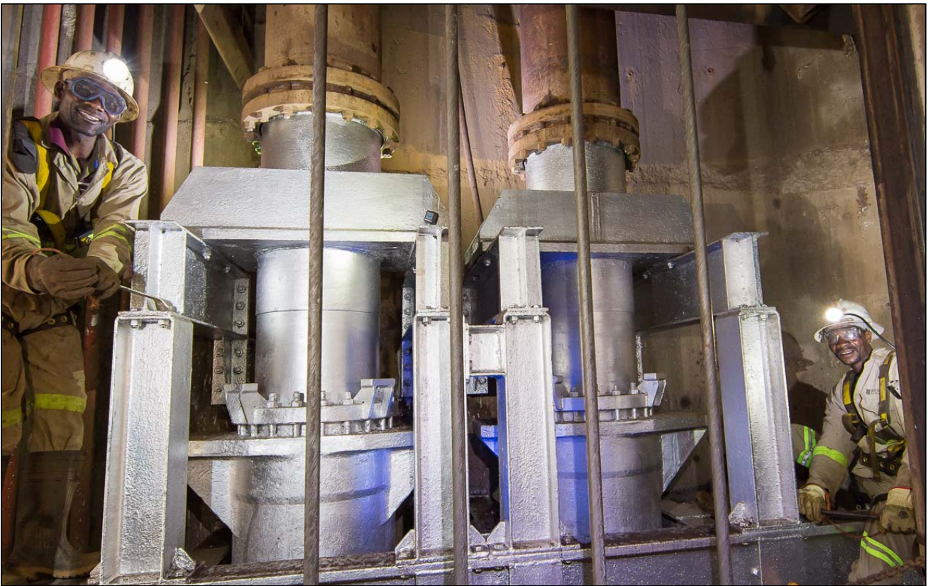
Figure 6: Upgraded supports for Shaft 5 pump columns at the 1,200-metre-level pump station.
