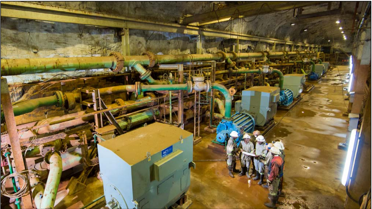
Figure 4: Shaft 5 main pumping station at the 1,200-metre level.
