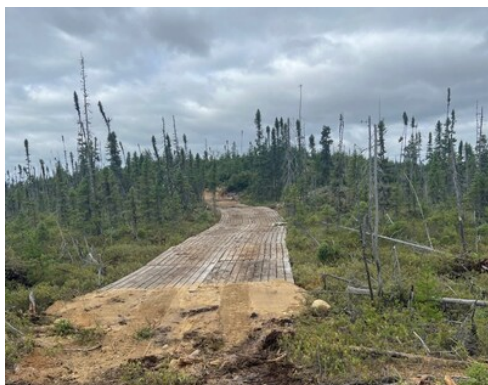
Figure 3: New drill road construction to access the Lion area all year round. (CNW Group/Power Metallic Mines Inc.)
