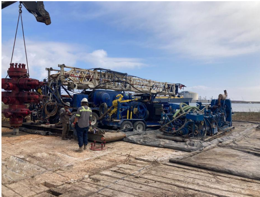
Cameron Parish, Louisiana: P&G Crew Members are Pictured Staging Equipment After Completing One Well and Before Moving to the Next Well Site
