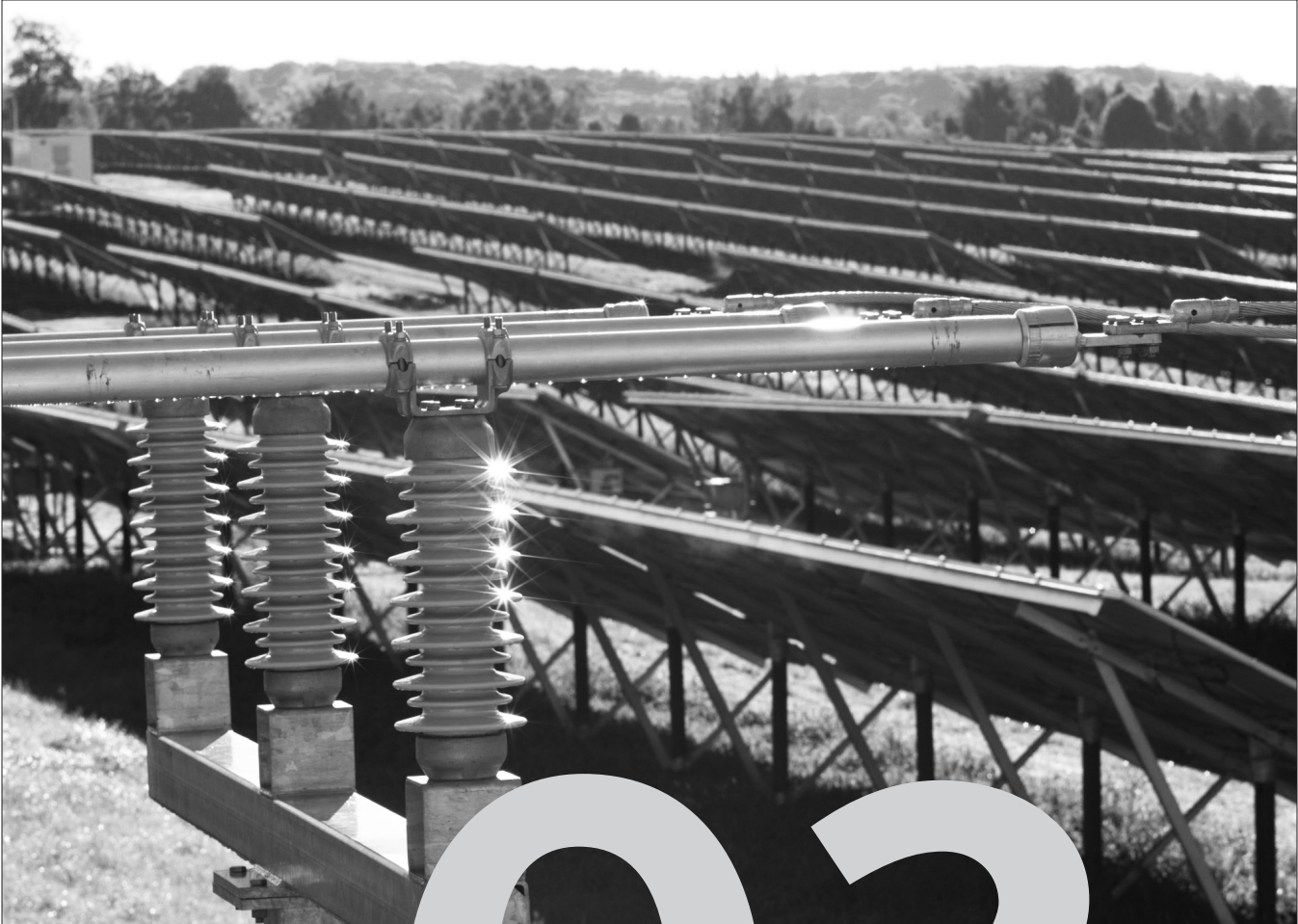
Grid line and panel arrays at Burk's Falls solar farm
