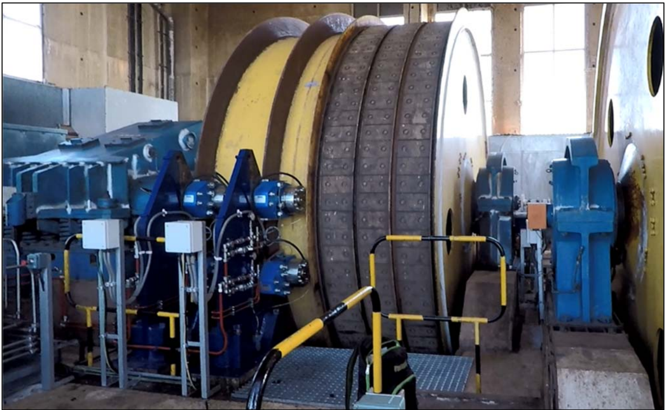
Figure 5: The fully-commissioned rock winder. All of the rock winder's safety and drive systems have been successfully tested to international standards.
