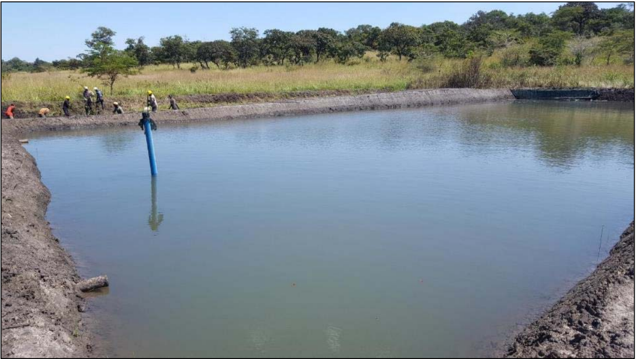
Figure 13: Construction of a new fish pond at one of the local villages, near the Kamoia-Kakula Project, as part of the project's community initiatives.
