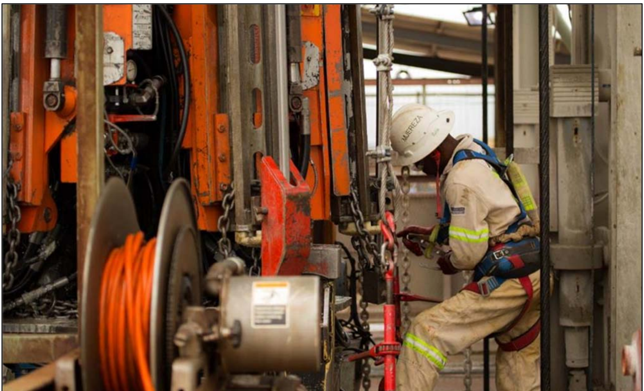
Figure 1: Jerry Molongama, a contract employee from Aveng Mining, securing the jumbo drilling rig on surface at Shaft 1. Construction of the station at the 750-metre level now is underway to provide initial mine development access to the orebody.
