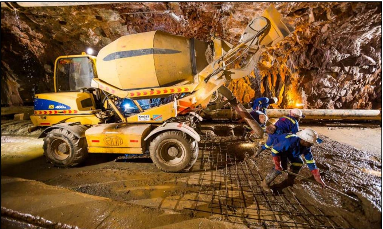
Figure 4: Pouring concrete for the new roadway on Kipushi's main haulage way at the 1,150-metre level.
