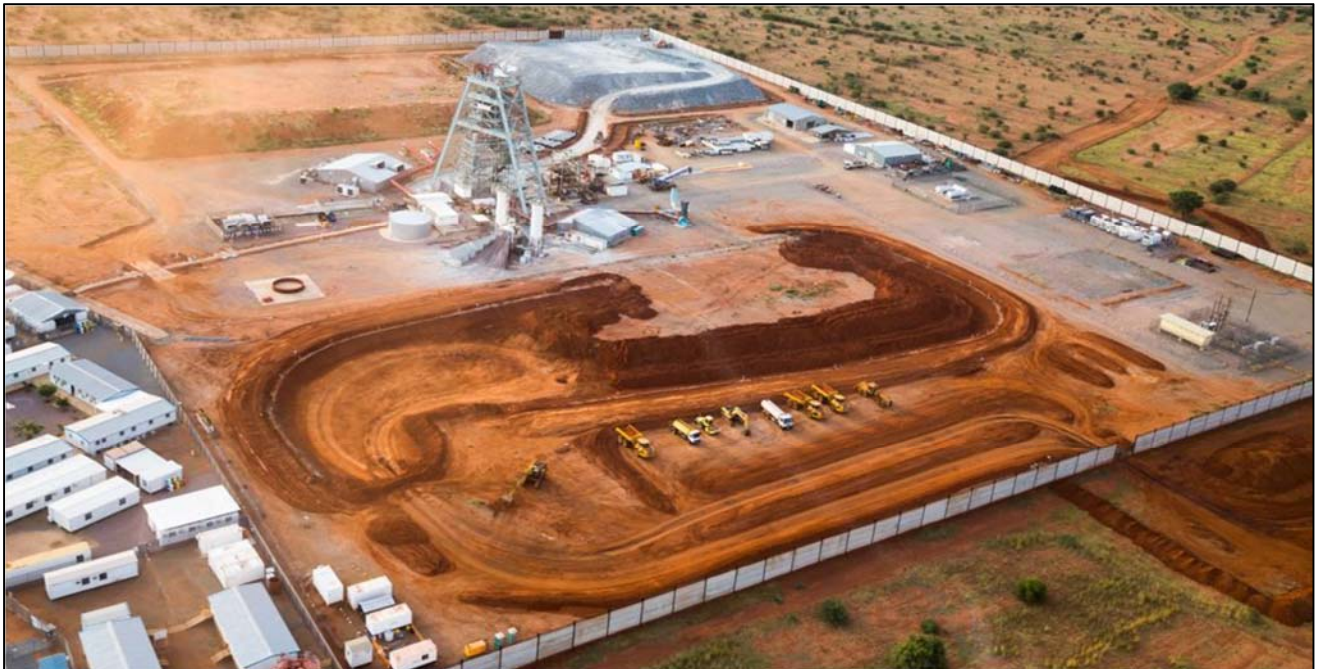
Figure 2: Excavation of a surface box cut now underway as part of early-works construction for Shaft 2 at the Platreef Mine in South Africa.
