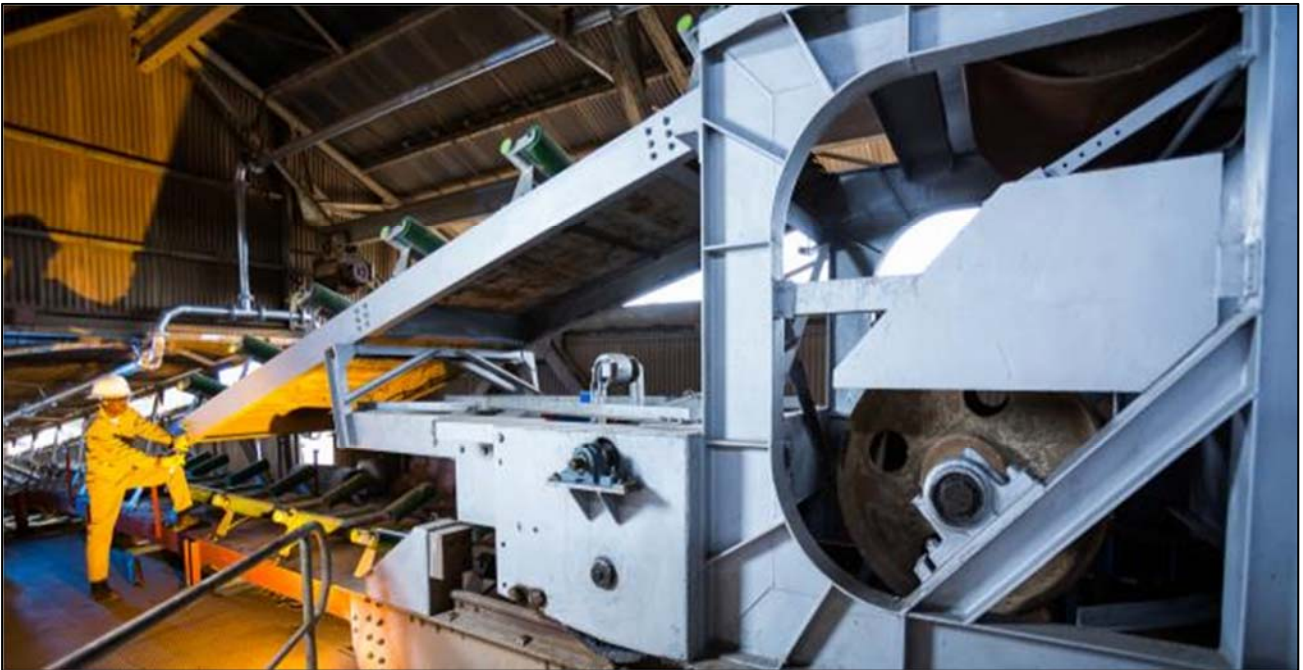
Figure 4: The new ore conveyor belt installed as part of Kipushi's upgrading work.
