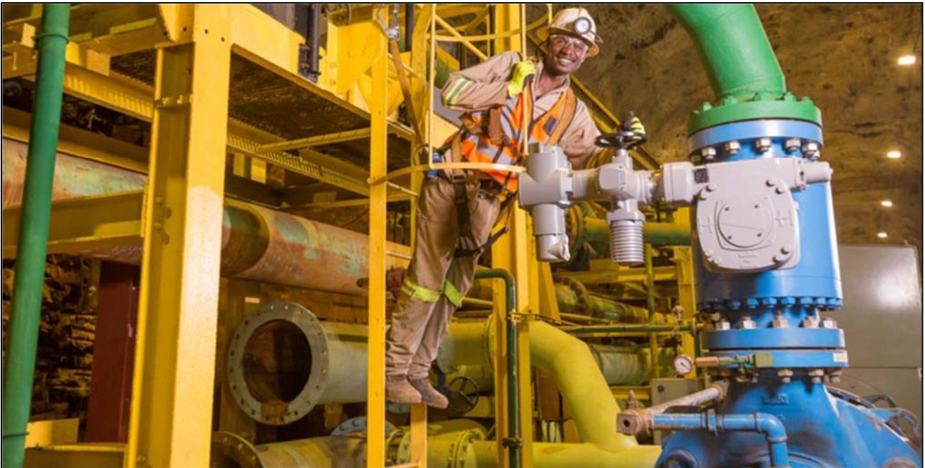
Figure 6: Shaft 5 main pumping station at Kipushi's 1,200-metre level.
