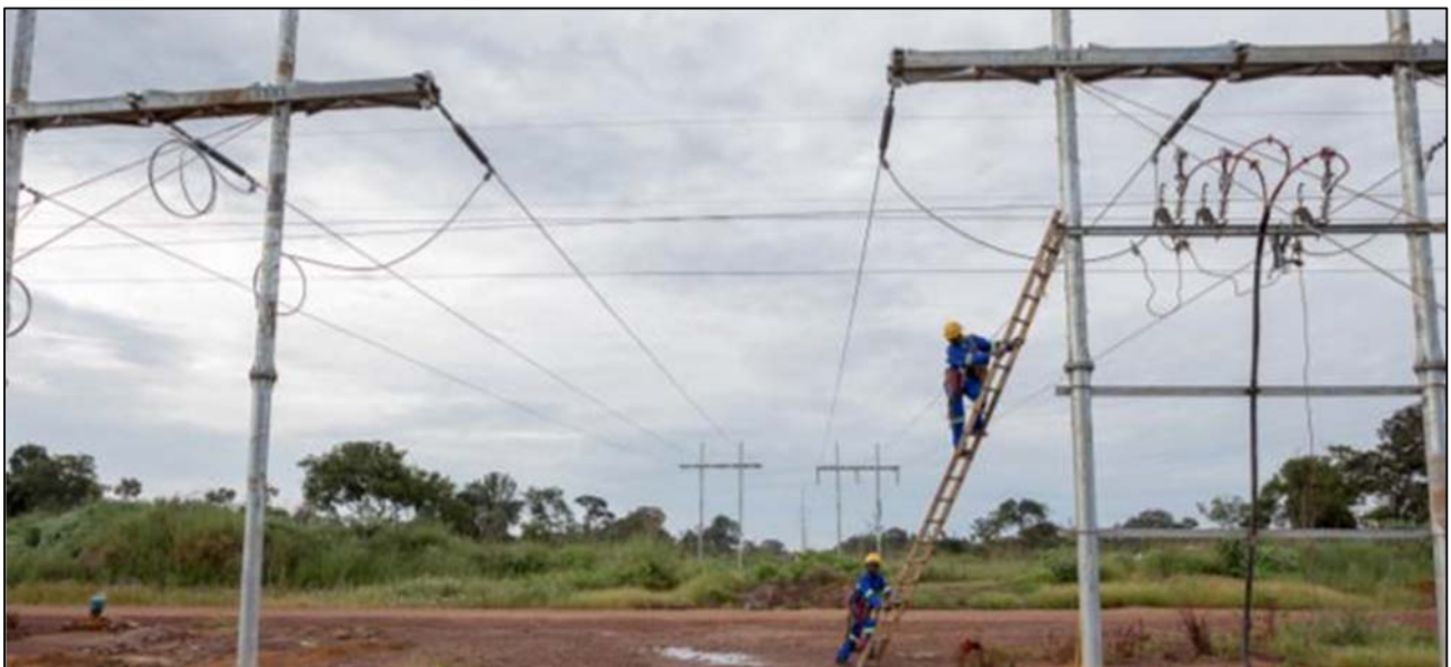
Figure 14: 120kV power line at the Kamoia-Kakula Project.
