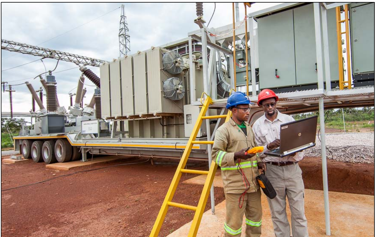
Figure 9: Kamoia mobile substation.
